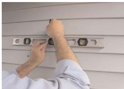
DRILL (4) 1/2" CORNER HOLES THROUGH WALL AND CONNECT HOLES ON EXTERIOR WITH A LEVEL.
